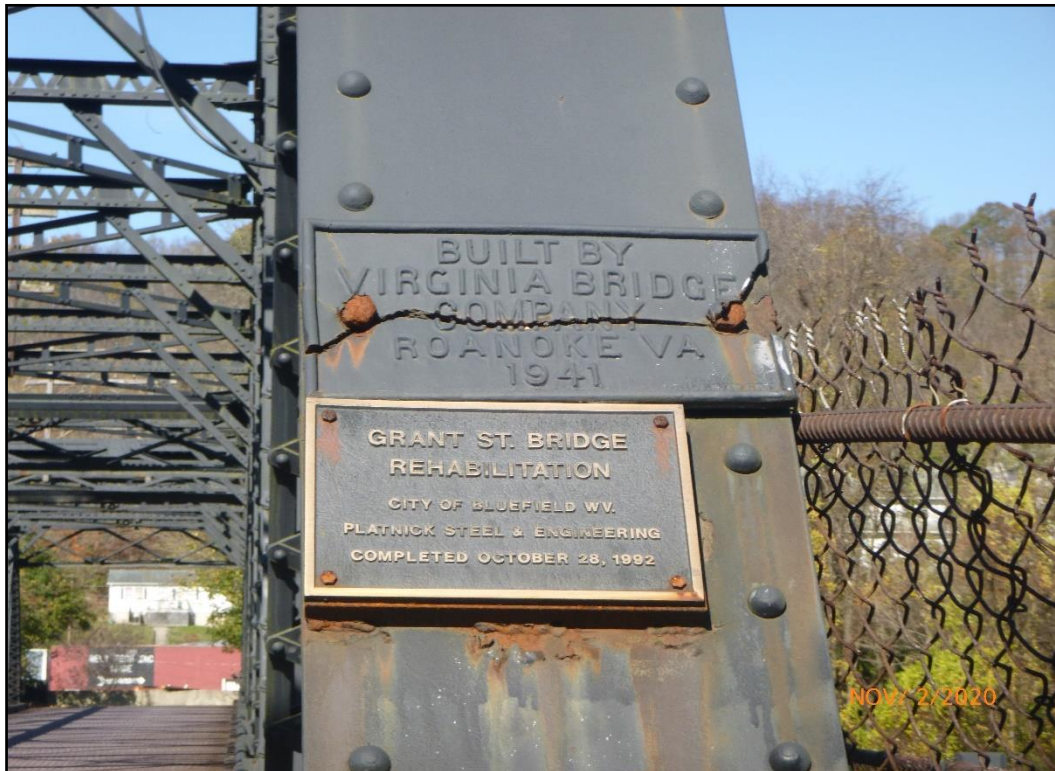
5. Detail of plaques. Photo: WVDOH November 2020.
