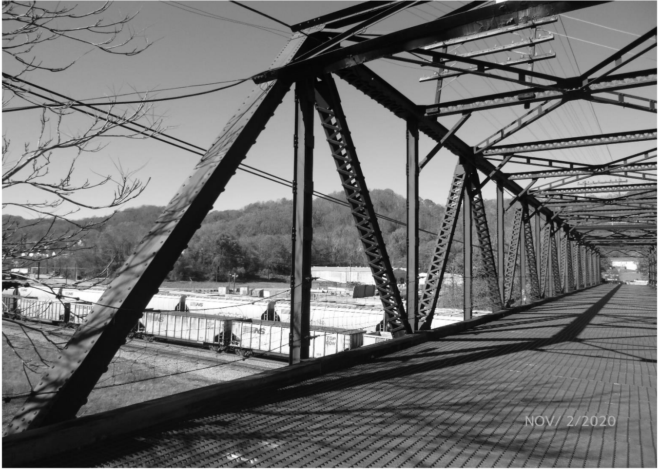
Photo 6 Grant Street Bridge City of Bluefield, Mercer County Grant Street over Norfolk Southern Railyard West elevation vertical and diagonal members
