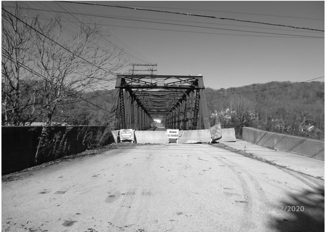
Photo 1 Grant Street Bridge City of Bluefield, Mercer County Grant Street over Norfolk Southern Railyard View northwest toward Grant Street Bridge
