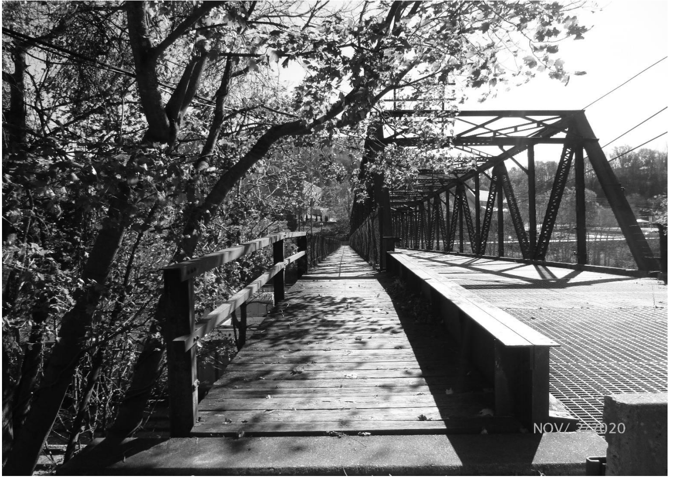
Photo 9 Grant Street Bridge City of Bluefield, Mercer County Grant Street over Norfolk Southern Railyard Wood plank sidewalk on east elevation
