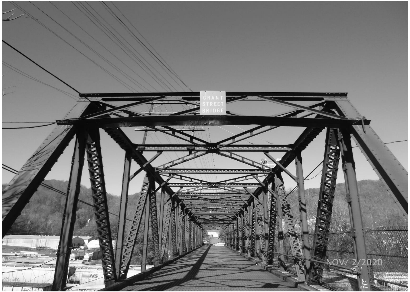
Photo 5 Grant Street Bridge City of Bluefield, Mercer County Grant Street over Norfolk Southern Railyard View of struts and laterals
