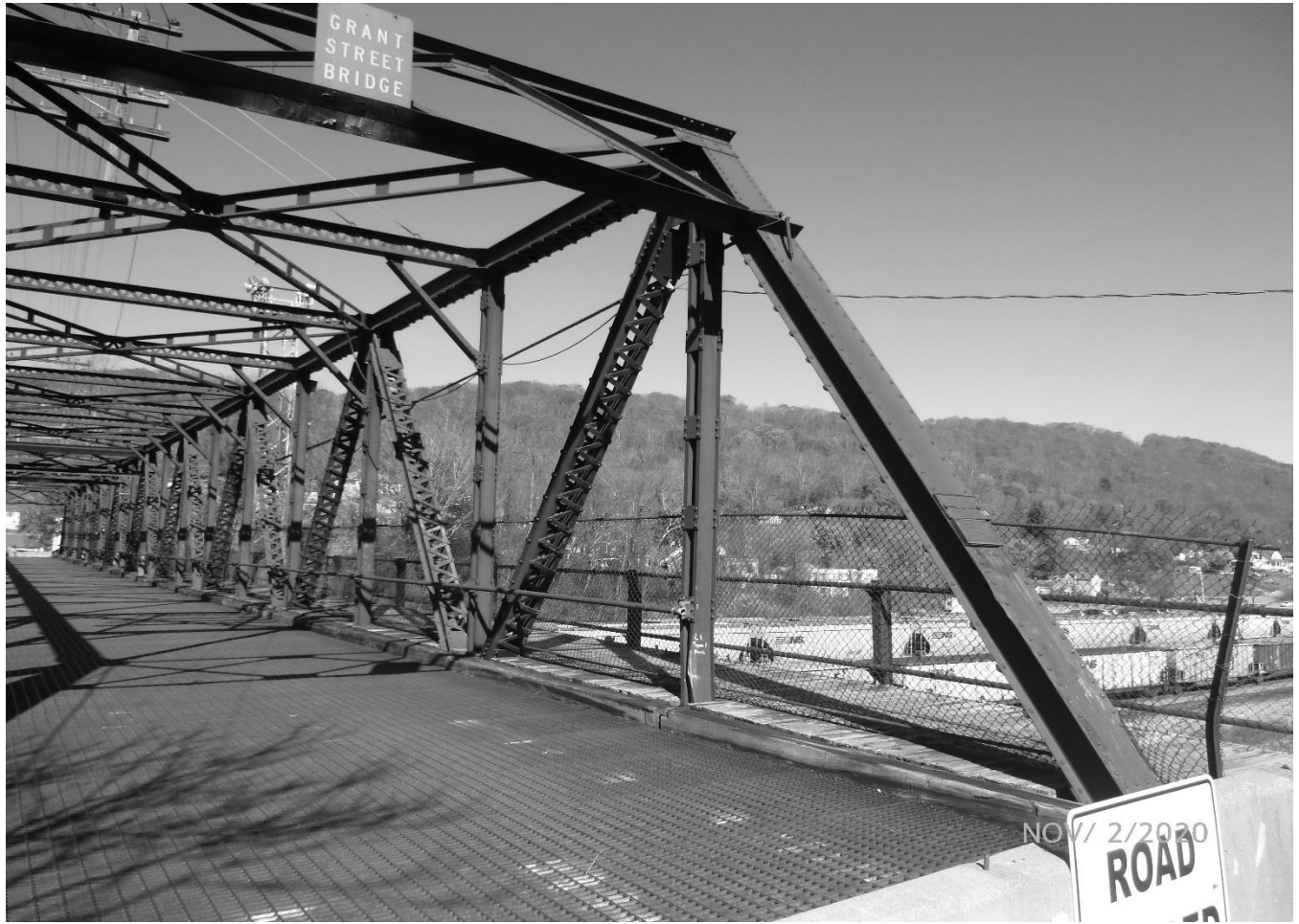
Photo 7 Grant Street Bridge City of Bluefield, Mercer County Grant Street over Norfolk Southern Railyard East elevation vertical and diagonal members
