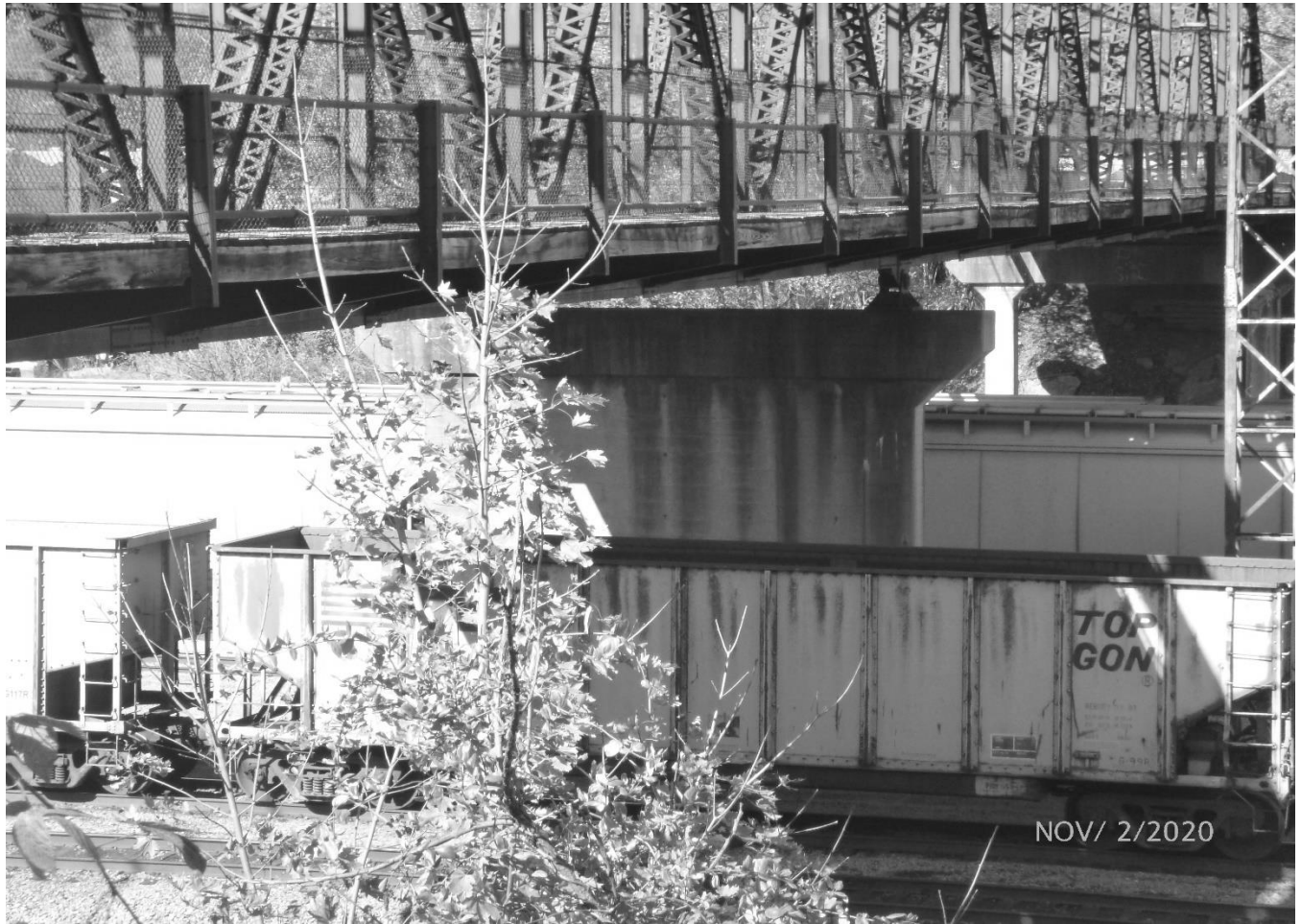
Photo 8 Grant Street Bridge City of Bluefield, Mercer County Grant Street over Norfolk Southern Railyard Pier and abutments in Norfolk Southern railyard
