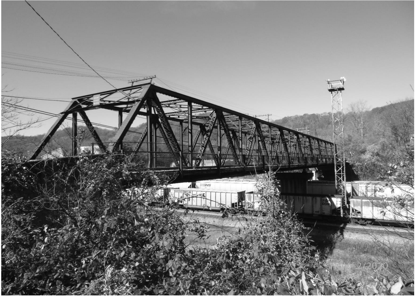
Photo 3 Grant Street Bridge City of Bluefield, Mercer County Grant Street over Norfolk Southern Railyard East elevation of Grant Street Bridge
