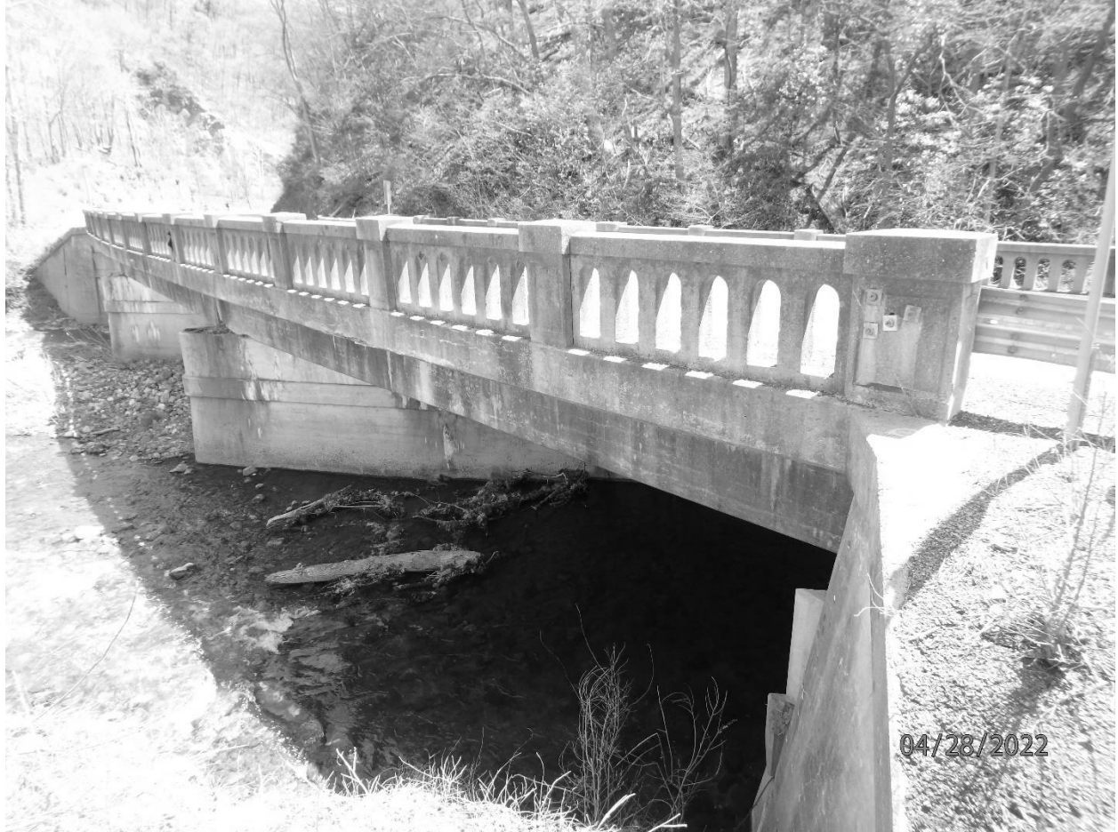
Photo #8 New Creek Bridge Mineral County US Route 50, spanning New Creek Looking east at downstream parapet
