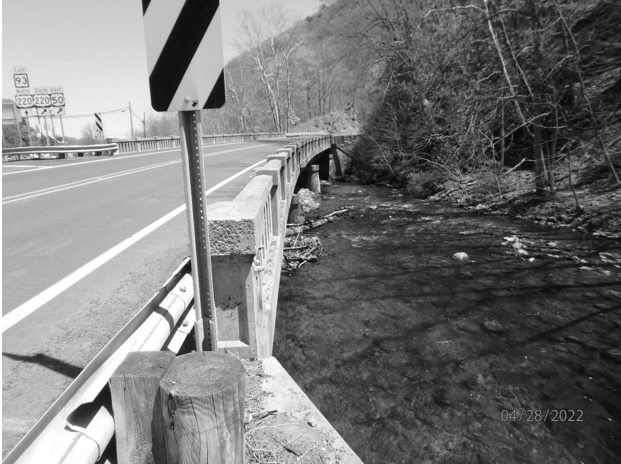
Photo #3 New Creek Bridge Mineral County US Route 50, spanning New Creek Looking east at upstream parapet
