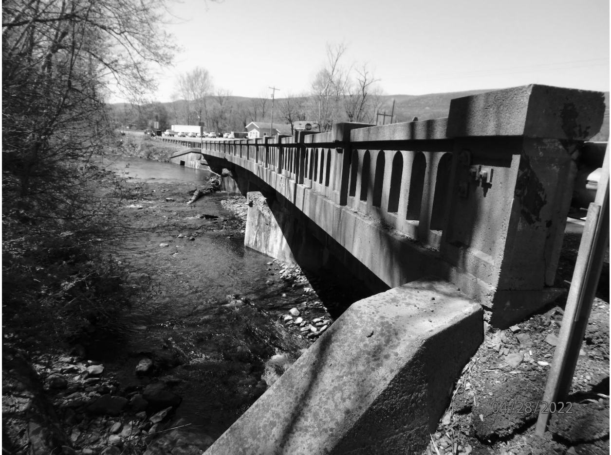
Photo #7 New Creek Bridge Mineral County US Route 50, spanning New Creek Looking west at upstream parapet
