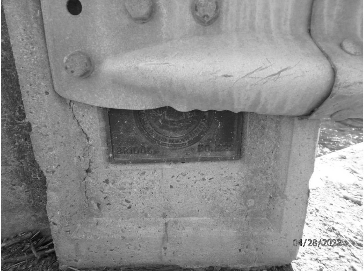
Photo #9 New Creek Bridge Mineral County US Route 50, spanning New Creek Looking at bridge plaque on south side of abutment 2
