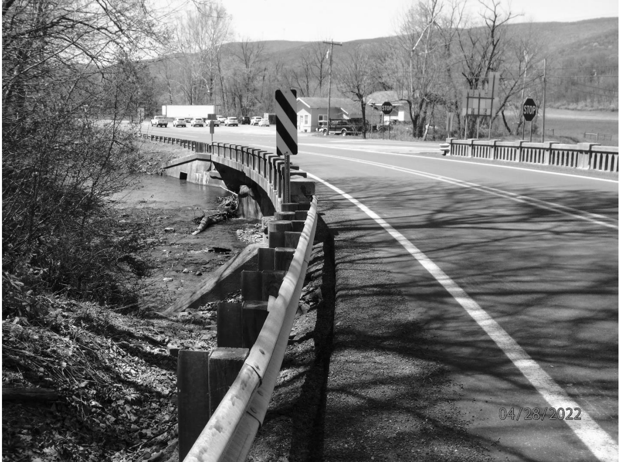
Photo #6 New Creek Bridge Mineral County US Route 50, spanning New Creek Looking west at New Creek Bridge
