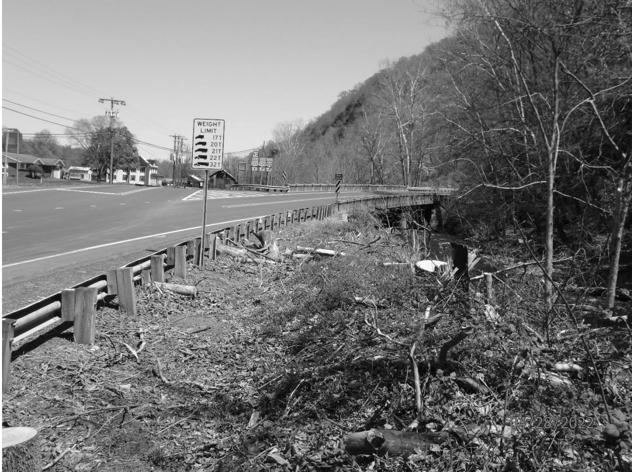
Photo #2 New Creek Bridge Mineral County US Route 50, spanning New Creek Looking east at New Creek Bridge
