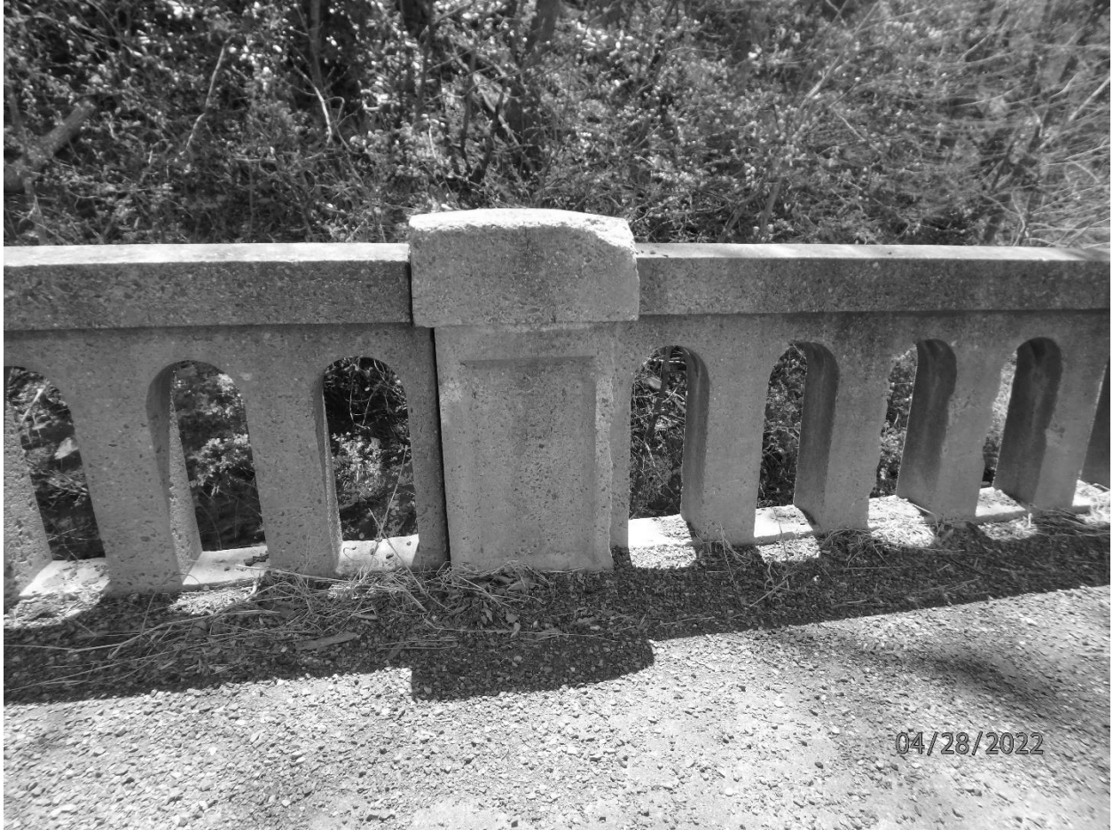
Photo #10 New Creek Bridge Mineral County US Route 50, spanning New Creek Looking at pierced parapet detail
