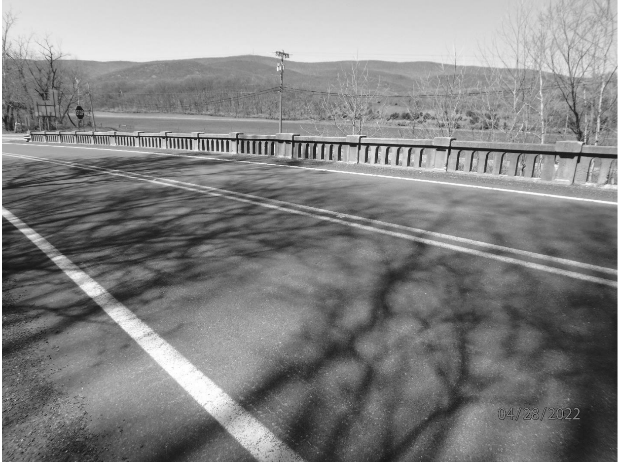
Photo #5 New Creek Bridge Mineral County US Route 50, spanning New Creek Looking at downstream parapet
