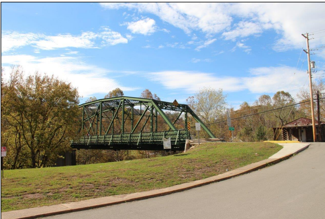
Photo 6. OBLIQUE VIEW OF NORTHEAST APPROACH OF BRIDGE FROM POWELL STREET, FACING WEST (WV_Gilmer County_Glenville Truss Bridge_0006).
