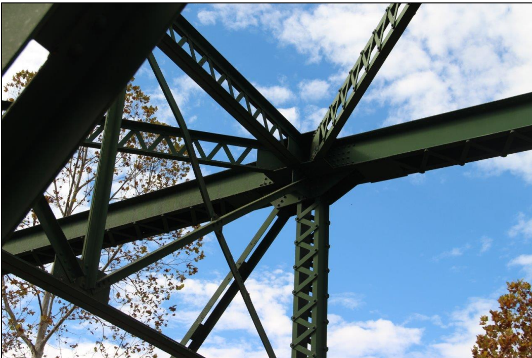
Photo 14. DETAIL OF UPPER CHORD, LATERAL BRACING, SWAY BRACING, AND VERTICAL POST OF NORTHWEST ELEVATION OF SPAN 2 (NORTHEAST), FACING NORTHWEST (WV_Gilmer County_Glenville Truss Bridge_0014).
