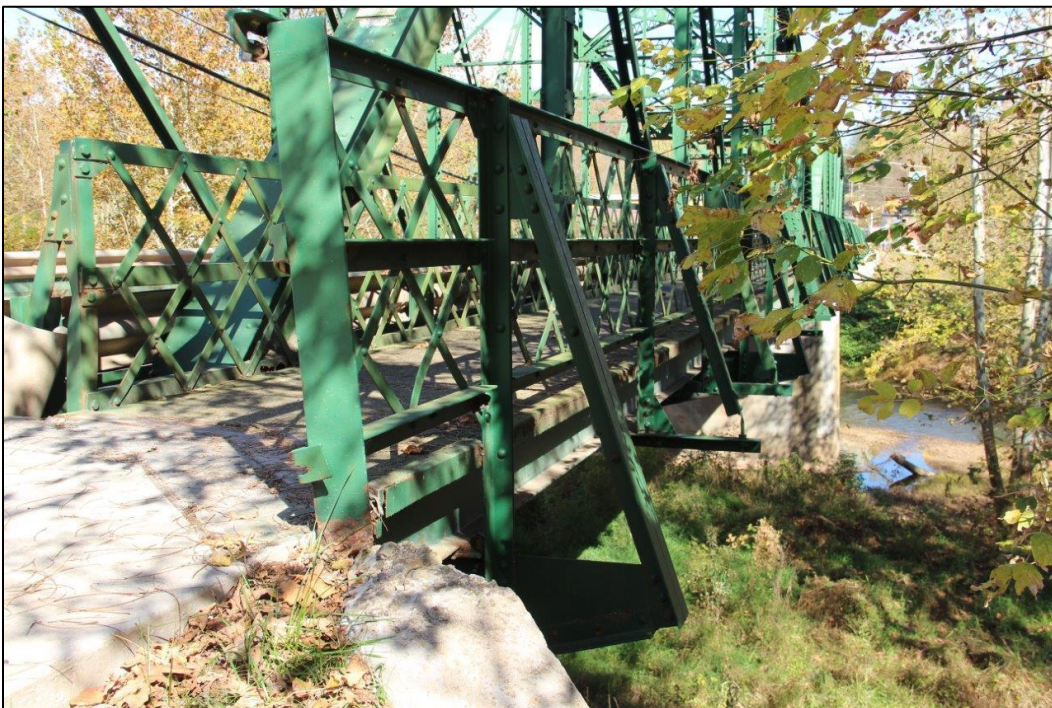
Photo 16. VIEW OF SOUTHEAST ELEVATION OF BRIDGE SHOWING SIDEWALK, RAILING AND BRACKET, FACING NORTHEAST (WV_Gilmer County_Glenville Truss Bridge_0016).
