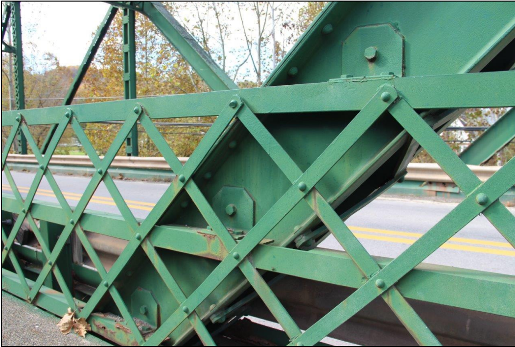
Photo 19. DETAIL OF LATTICE RAILING AND BOTTOM OF INCLINED END POST AT SOUTHWEST END OF SPAN 2 (NORTHEAST), FACING WEST (WV_Gilmer County_Glenville Truss Bridge_0019).
