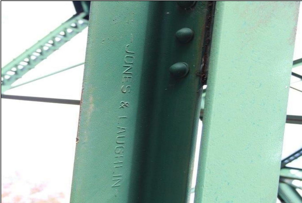
Photo 35. DETAIL OF JONES AND LAUGHLIN STEEL COMPANY MARKING ON SOUTHEAST ELEVATION OF SPAN 1 (SOUTHWEST) TRUSS, FACING NORTH (WV_Gilmer County_Glenville Truss Bridge_0035).
