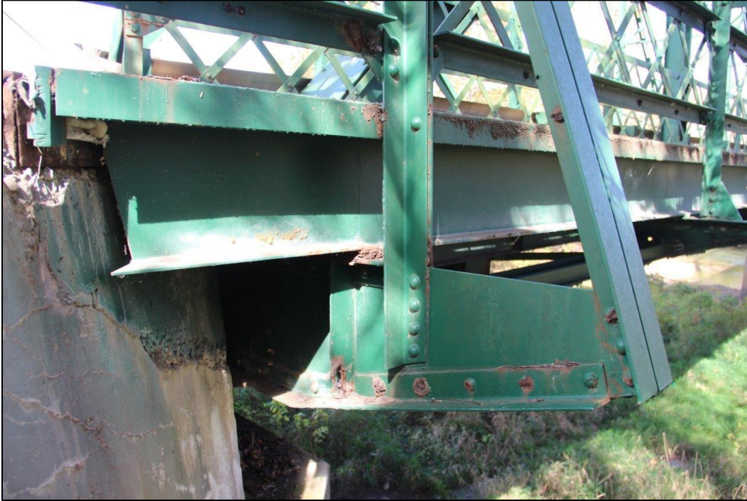
Photo 17. DETAIL VIEW OF SIDEWALK BRACKET, FASCIA BEAM, AND SOUTHWEST ABUTMENT, FACING NORTH (WV_Gilmer County_Glenville Truss Bridge_0017).
