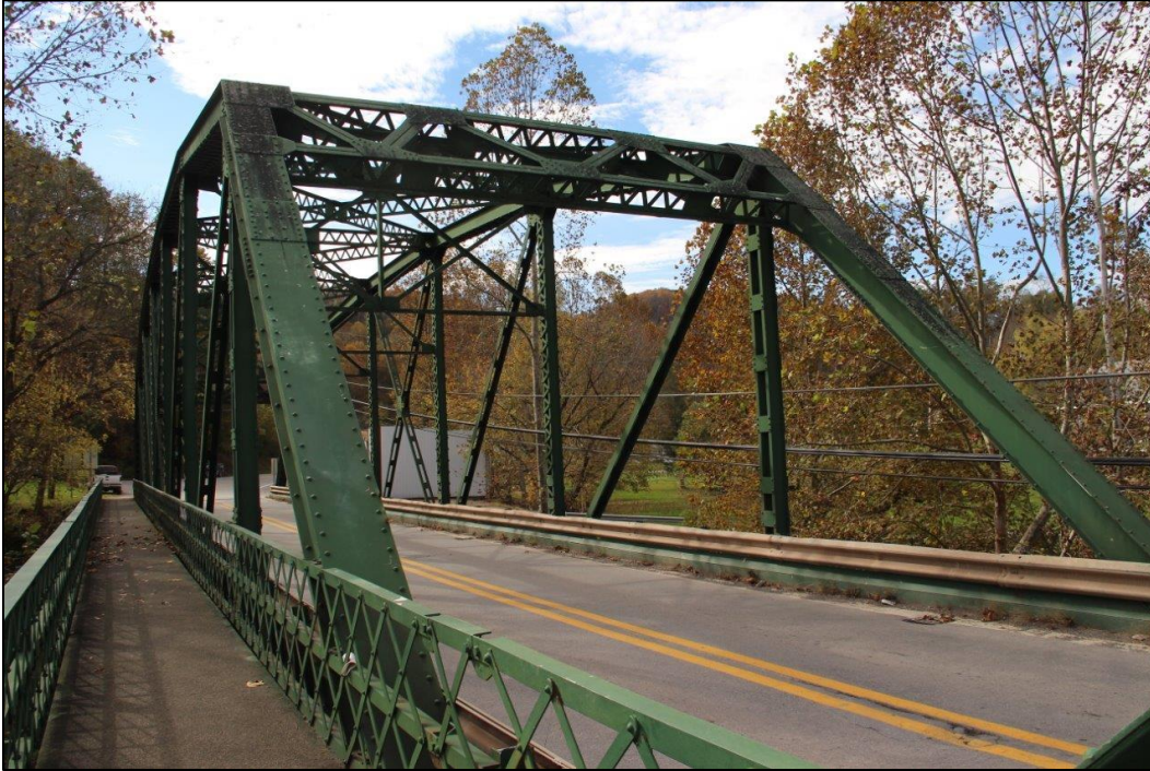
Photo 9. DETAIL OF SIDEWALK, NORTHEAST END POSTS, AND ROAD DECK OF SPAN 1 (SOUTHWEST), FACING SOUTHWEST (WV_Gilmer County_Glenville Truss Bridge_0009).
