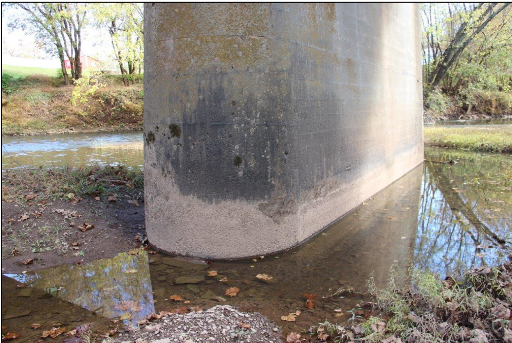
Photo 26. DETAIL OF NORTHWEST AND SOUTHWEST SIDES OF PIER, FACING EAST (WV_Gilmer County_Glenville Truss Bridge_0026).
