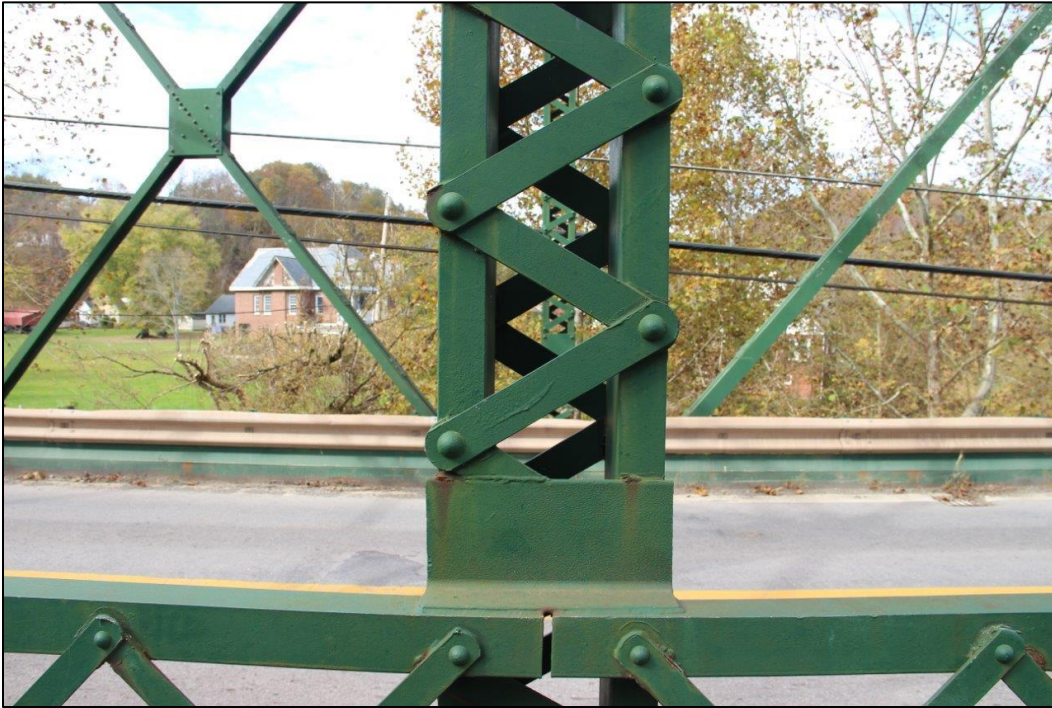
Photo 21. DETAIL OF VERTICAL IN THE CENTER OF SPAN 1 (SOUTHWEST), FACING NORTHWEST (WV_Gilmer County_Glenville Truss Bridge_0021).
