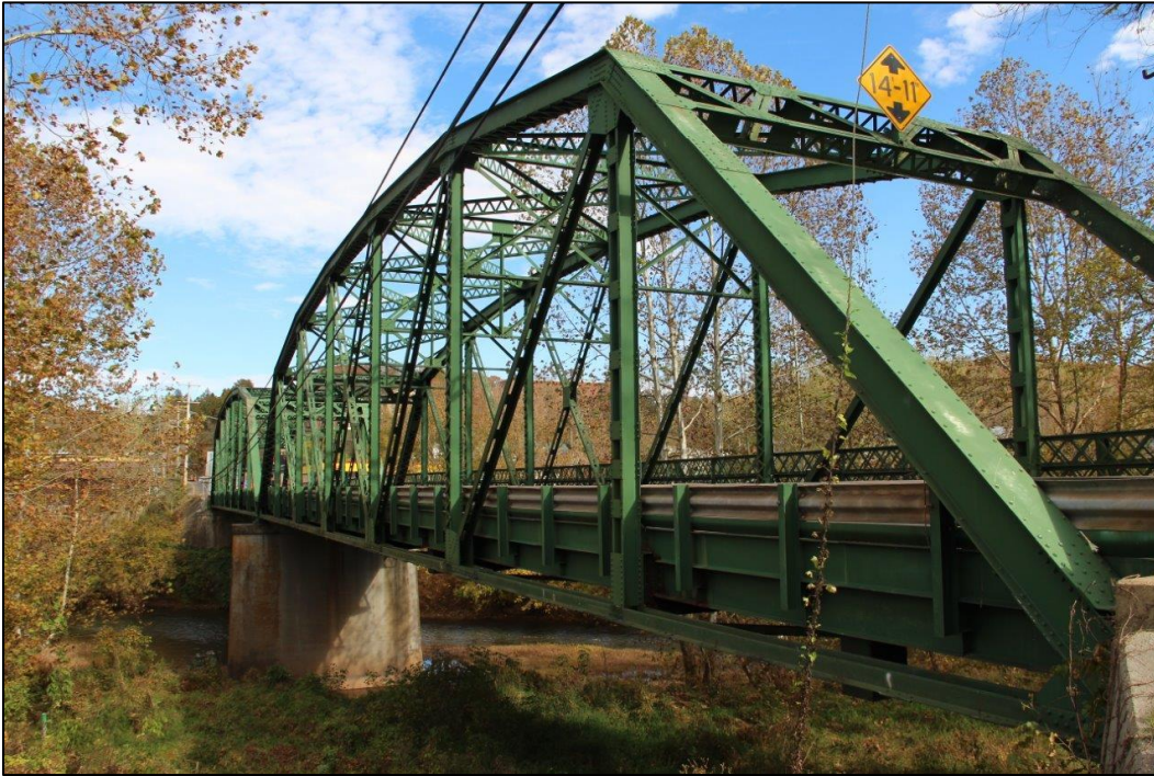
Photo 7. OBLIQUE VIEW OF NORTHWEST ELEVATION OF BRIDGE, FACING EAST (WV_Gilmer County_Glenville Truss Bridge_0007).
