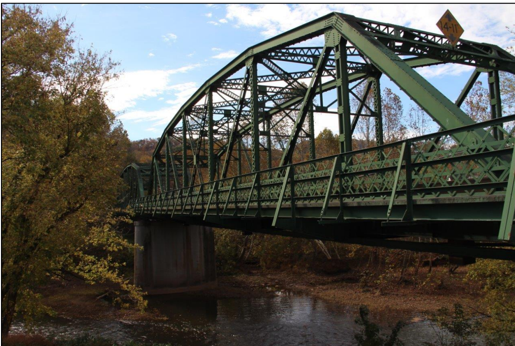
Photo 4. OBLIQUE VIEW OF SOUTHEAST ELEVATION OF BRIDGE, FACING WEST (WV_Gilmer County_Glenville Truss Bridge_0004).
