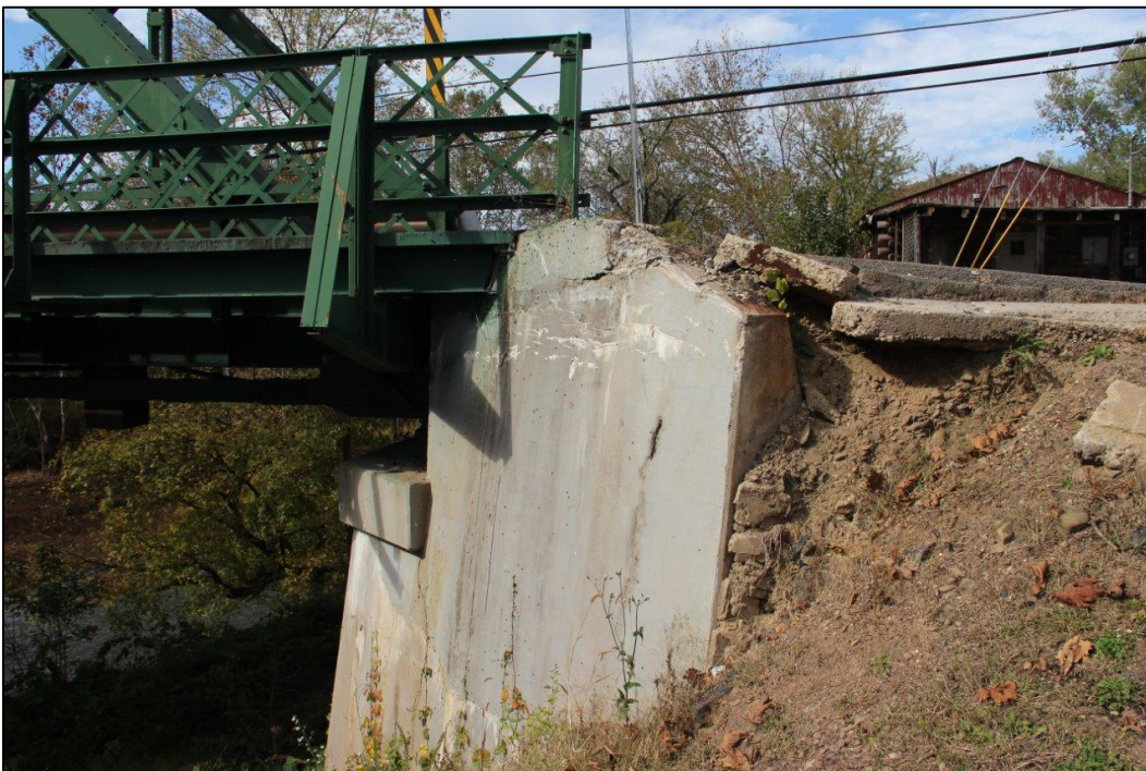
Photo 32. DETAIL OF SOUTHEAST WINGWALL OF NORTHEAST ABUTMENT, FACING NORTHWEST (WV_Gilmer County_Glenville Truss Bridge_0032).
