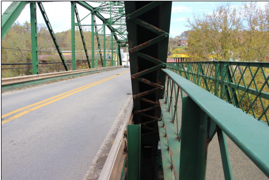
Photo 12. DETAIL OF LATTICE BRACING ON UNDERSIDE OF END POST OF NORTHEAST PORTAL OF SPAN 1 (SOUTHWEST), FACING NORTHEAST (WV_Gilmer County_Glenville Truss Bridge_0012).
