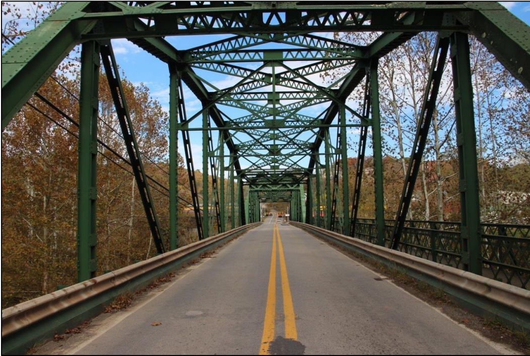
Photo 3. VIEW OF ROADWAY AND THROUGH TRUSS FROM SOUTHWEST END OF BRIDGE, FACING NORTHEAST (WV_Gilmer County_Glenville Truss Bridge_0003).
