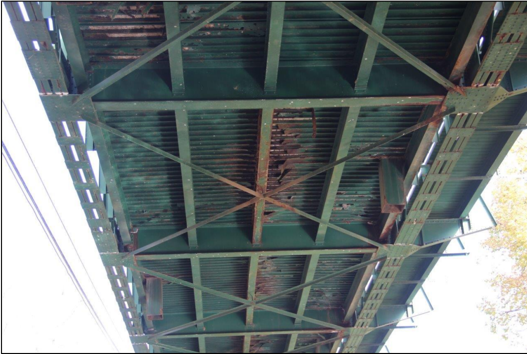
Photo 27. UNDERSIDE OF SPAN 1 (SOUTHWEST), SHOWING LOWER CHORDS, FLOOR BEAMS, STRINGERS, AND LOWER LATERAL BRACING, FACING NORTHEAST (WV_Gilmer County_Glenville Truss Bridge_0027).
