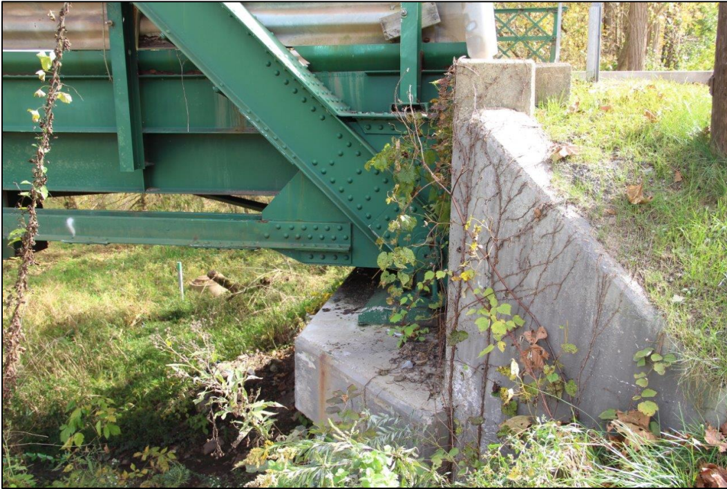
Photo 31. DETAIL OF NORTHWEST WINGWALL OF SOUTHWEST ABUTMENT, SHOWING BOTTOM OF END POST, BRIDGE SEAT, AND BEARING, FACING SOUTHEAST (WV_Gilmer County_Glenville Truss Bridge_0031).
