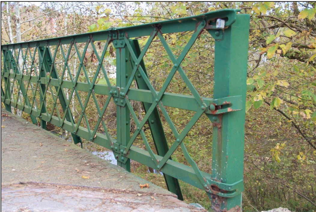
Photo 18. DETAIL OF SIDEWALK END POST AND LATTICE AT SOUTHWEST END OF BRIDGE, FACING EAST (WV_Gilmer County_Glenville Truss Bridge_0018).
