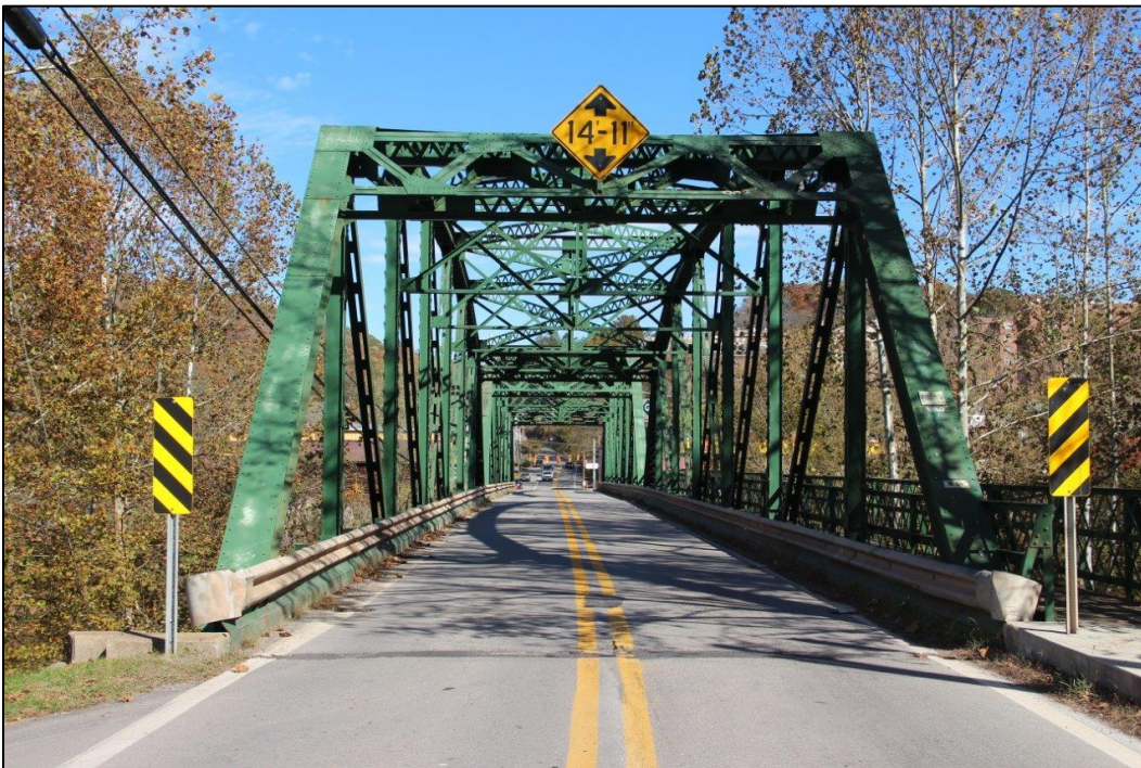
Photo 2. SOUTHWEST APPROACH TO BRIDGE FROM CENTER OF US 33/US 119, FACING NORTHEAST (WV_Gilmer County_Glenville Truss Bridge_0002).
