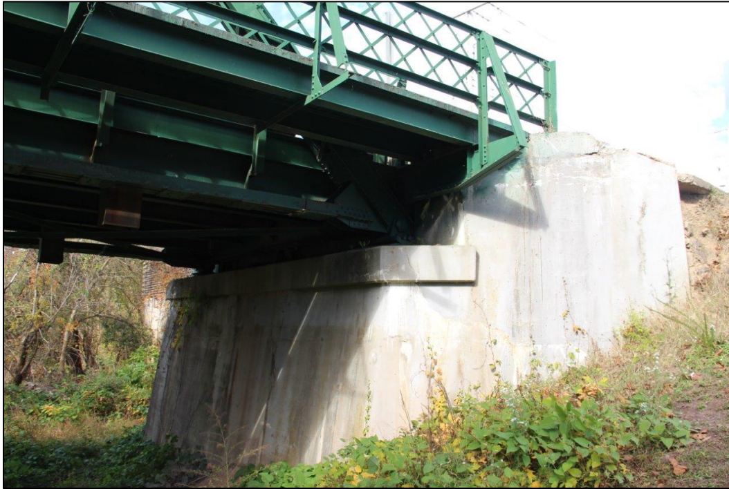
Photo 33. VIEW OF NORTHEAST ABUTMENT AND BRIDGE SEAT, FACING NORTH (WV_Gilmer County_Glenville Truss Bridge_0033).
