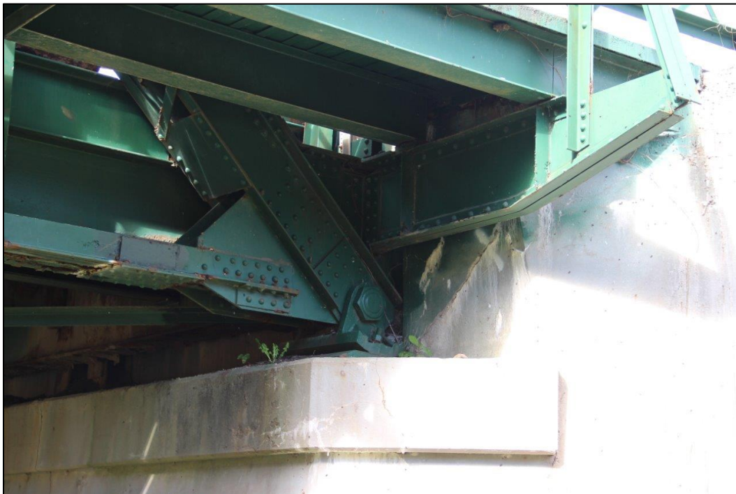
Photo 34. DETAIL OF NORTHEAST ABUTMENT, SHOWING BRIDGE SEAT AND BEARING WITH PINNED CONNECTION, FACING NORTH (WV_Gilmer County_Glenville Truss Bridge_0034).
