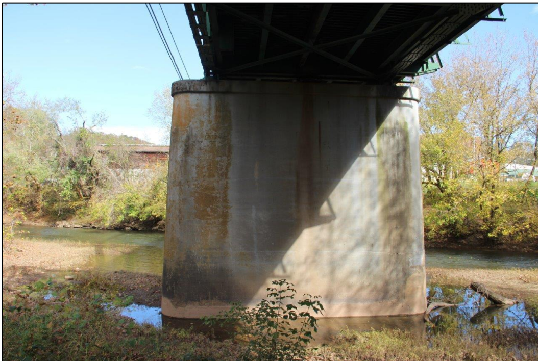
Photo 24. VIEW OF SOUTHWEST ELEVATION OF PIER, FACING NORTHEAST (WV_Gilmer County_Glenville Truss Bridge_0024).
