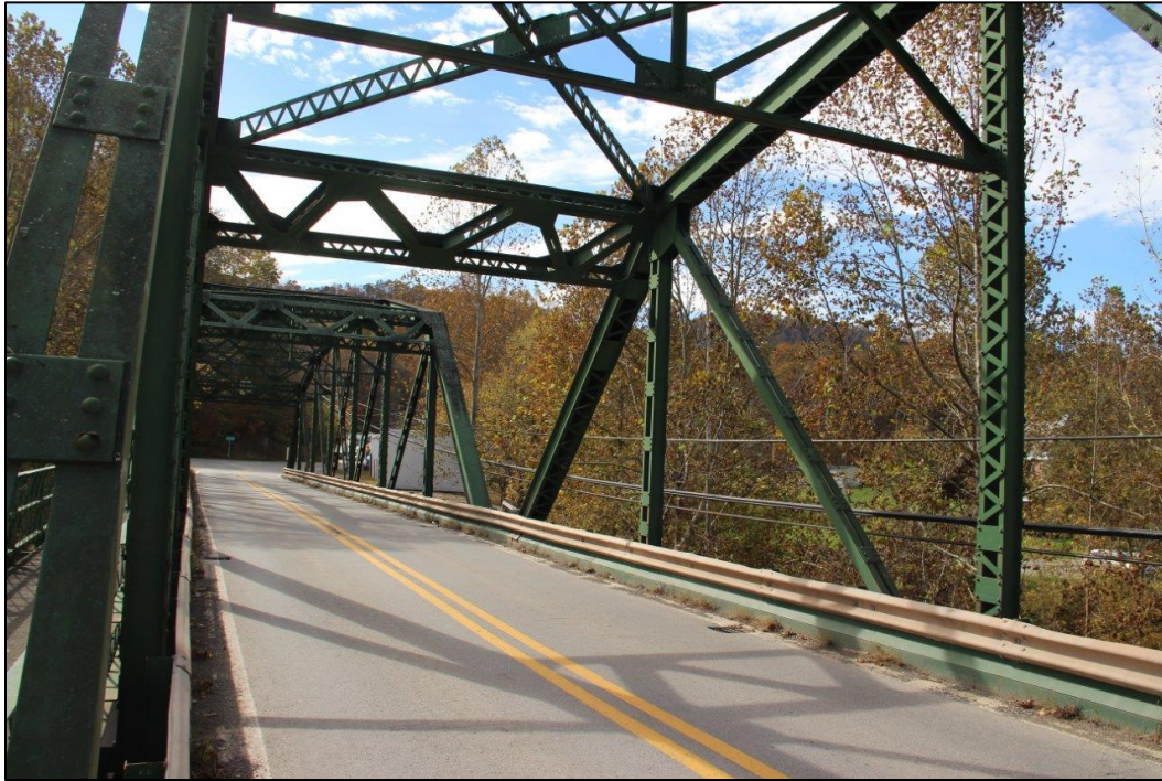
Photo 11. INTERIOR VIEW FROM THE END OF SPAN 2 SHOWING VERTICALS, DIAGONALS, CROSS BRACING, AND SOUTHWEST PORTAL OF SPAN 2 (NORTHEAST), FACING SOUTHWEST (WV_Gilmer County_Glenville Truss Bridge_0011).
