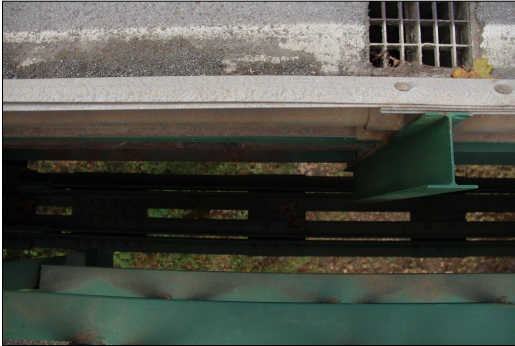
Photo 23. VIEW OF LOWER CHORD FROM SIDEWALK, FACING DOWN (WV_Gilmer County_Glenville Truss Bridge_0023).
