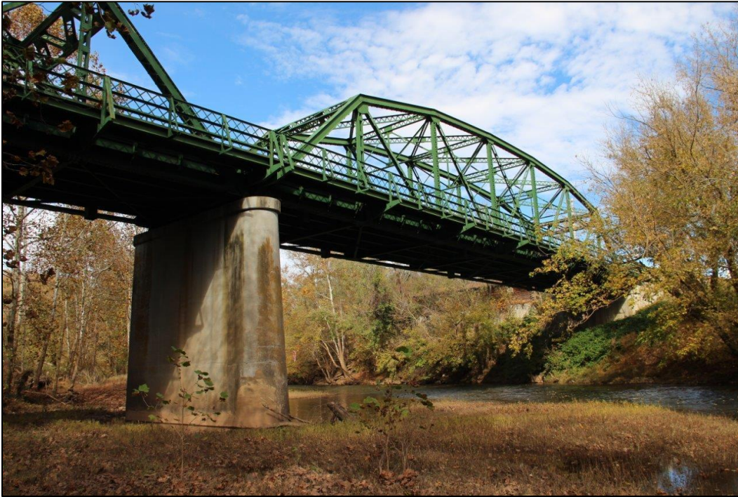
Photo 5. VIEW OF SOUTHEAST ELEVATION OF PIER AND BRIDGE FROM LITTLE KANAWHA RIVER, FACING NORTH (WV_Gilmer County_Glenville Truss Bridge_0005).
