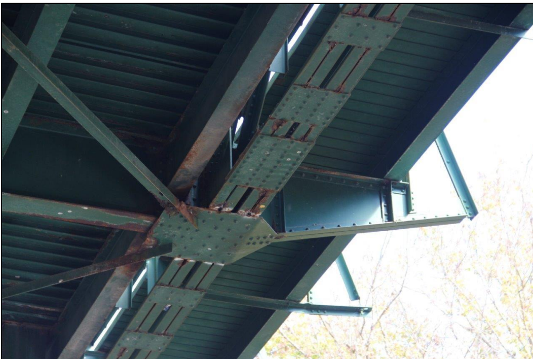
Photo 30. DETAIL VIEW OF GUSSET PLATE CONNECTING FLOORBEAM, SIDEWALK BRACKET, AND LOWER CHORD ON SOUTHEAST ELEVATION OF SPAN 1 (SOUTHWEST), FACING NORTHEAST (WV_Gilmer County_Glenville Truss Bridge_0030).
