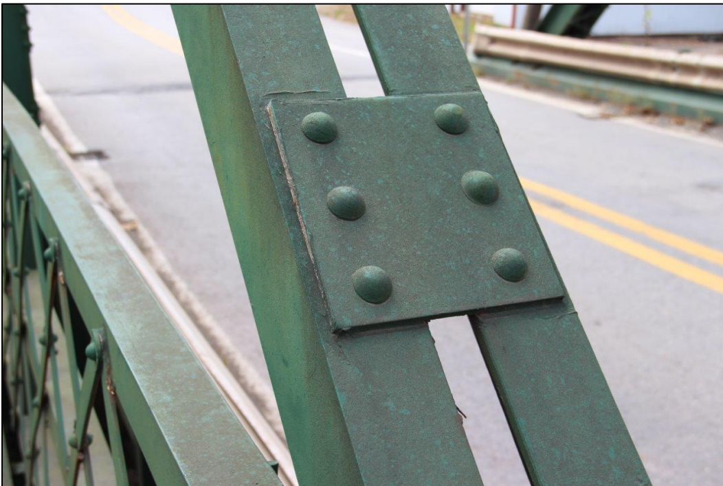
Photo 22. DETAIL OF DIAGONAL ON SOUTHEAST SIDE OF SPAN 1 (SOUTHWEST), FACING WEST (WV_Gilmer County_Glenville Truss Bridge_0022).
