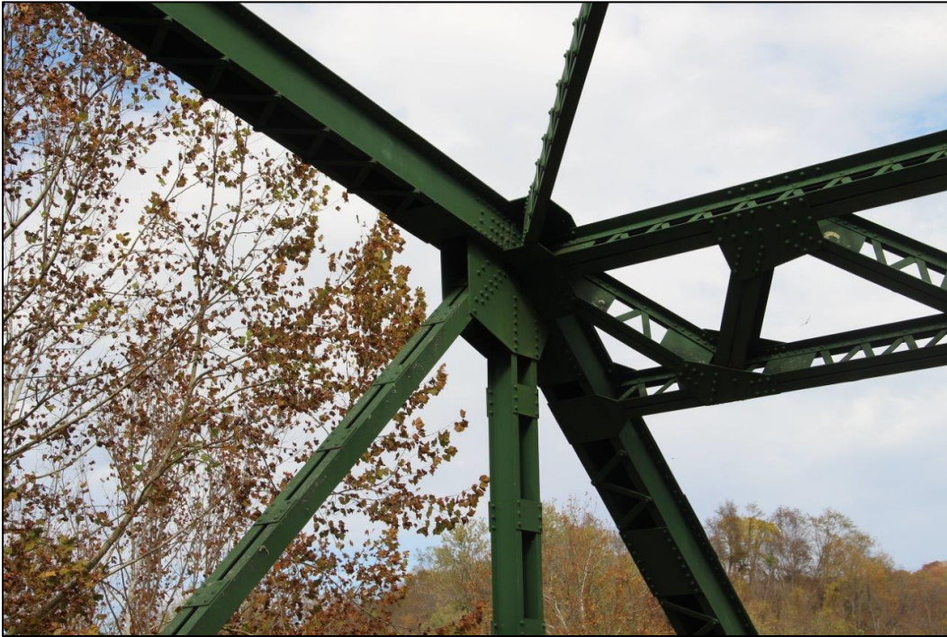
Photo 15. DETAIL OF INCLINED END POST, HIP VERTICAL, AND PORTAL BRACING OF NORTHEAST PORTAL OF SPAN 2 (NORTHEAST), FACING NORTH (WV_Gilmer County_Glenville Truss Bridge_0015).
