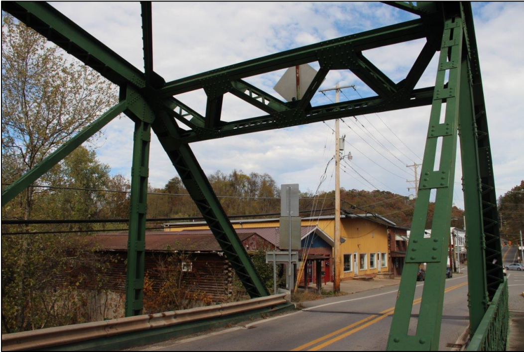
Photo 13. DETAIL OF NORTHEAST PORTAL OF SPAN 2 (NORTHEAST), FACING NORTHEAST (WV_Gilmer County_Glenville Truss Bridge_0013).
