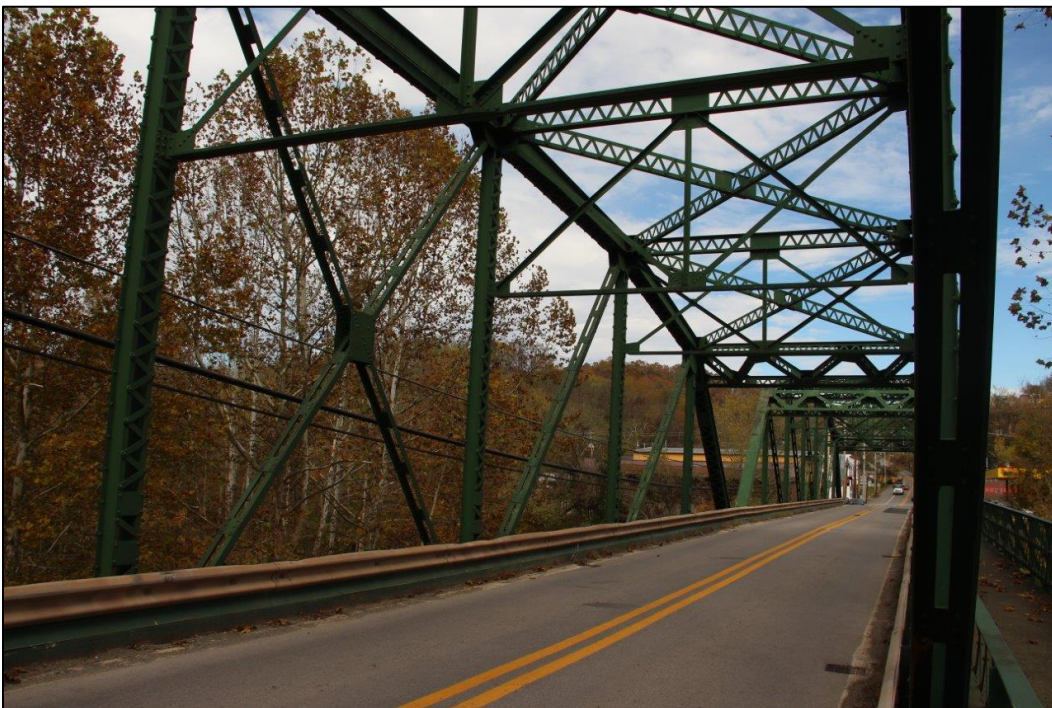
Photo 10. INTERIOR VIEW FROM MIDDLE OF SPAN 1 (SOUTHWEST) SHOWING ROAD DECK AND TRUSS DETAILS, FACING NORTHEAST (WV_Gilmer County_Glenville Truss Bridge_0010).
