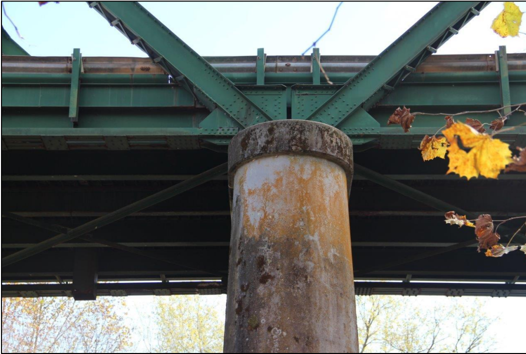
Photo 25. DETAIL OF NORTHWEST ELEVATION OF PIER AND INCLINED END POSTS OF SPANS 1 AND 2, FACING SOUTHEAST (WV_Gilmer County_Glenville Truss Bridge_0025).
