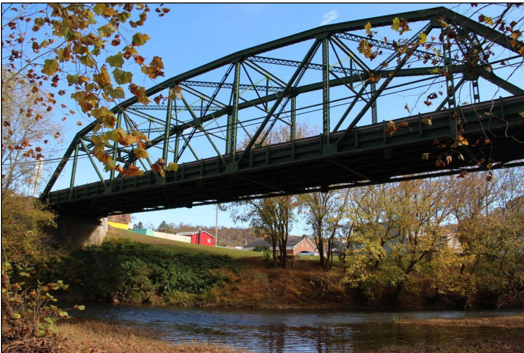
Photo 8. VIEW OF NORTHWEST ELEVATION OF SPAN 2 (NORTHEAST) FROM LITTLE KANAWHA RIVER, FACING EAST (WV_Gilmer County_Glenville Truss Bridge_0008).
