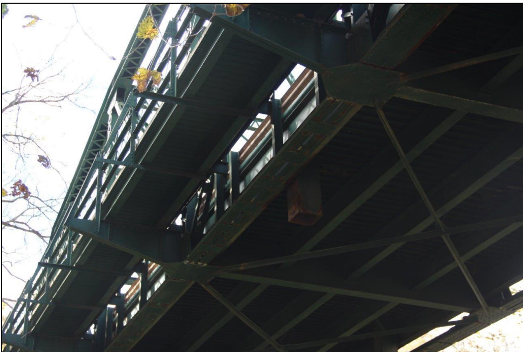
Photo 28. VIEW OF THE UNDERSIDE OF SPAN 1 (SOUTHWEST) SHOWING SIDEWALK, FLOOR BEAMS, STRINGERS, LATERAL BRACING, AND LOWER CHORD, FACING SOUTHWEST (WV_Gilmer County_Glenville Truss Bridge_0028).
