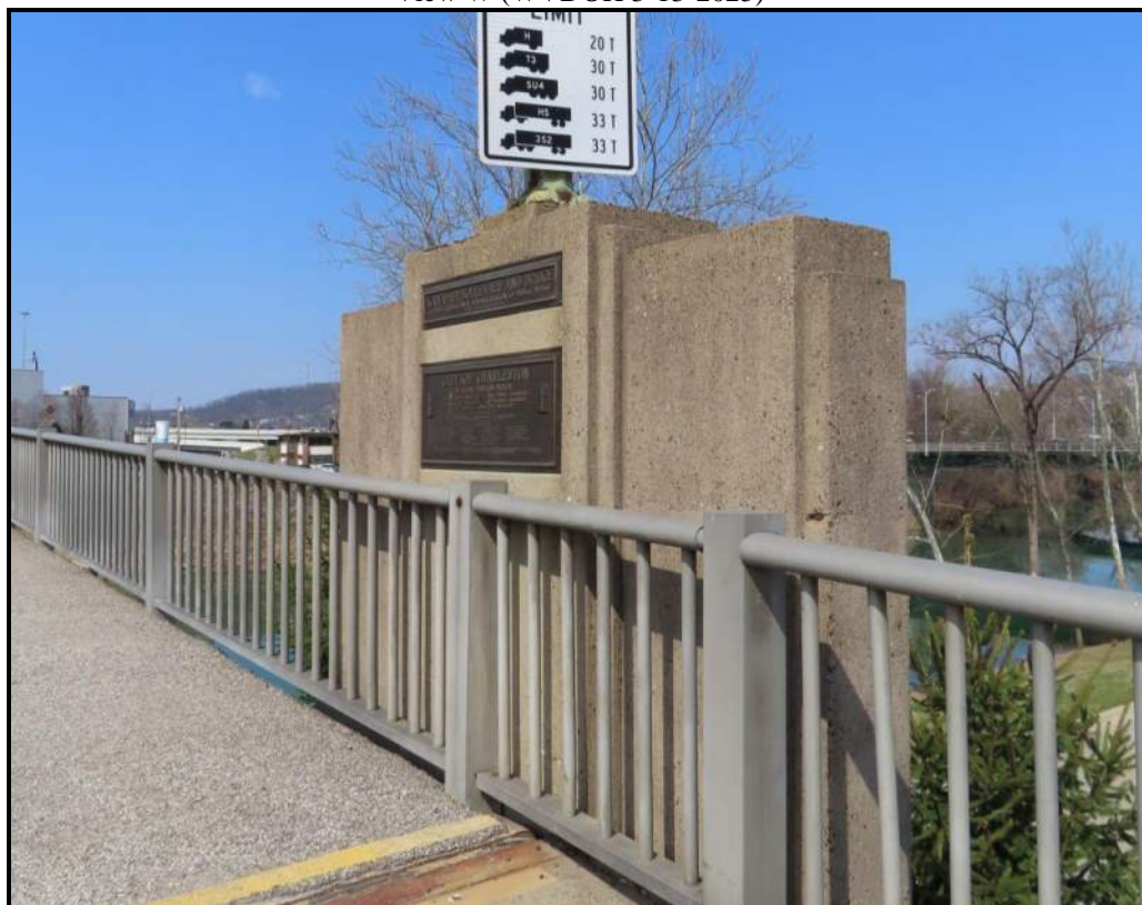
Pylon at East End, North/Upstream Side. Includes original 1930s plaques. View NNW (WVDOH 3-13-2025)
