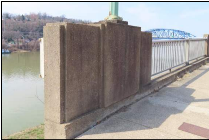
Typ. Partial Pylon at Ends of Return Wingwalls. Example is the South/Downstream East Partial Pylon. View WNW (WVDOH 3-13-2025)
