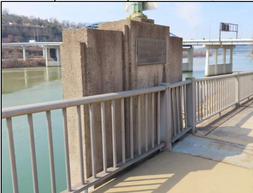
Pylon at West End, South/Downstream Side. Includes a 1980s plaque. View W (WVDOH 3-13-2025)
