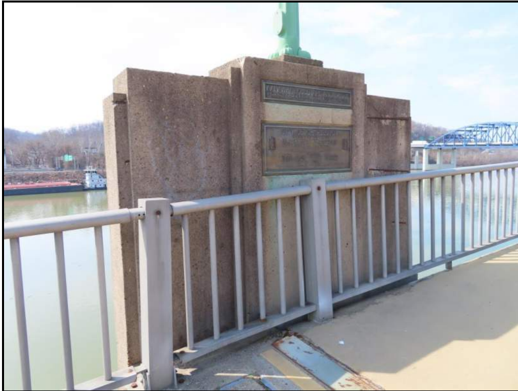
Pylon at East End, South/Downstream Side. Includes original 1930s plaques. View W (WVDOH 3-13-2025)
