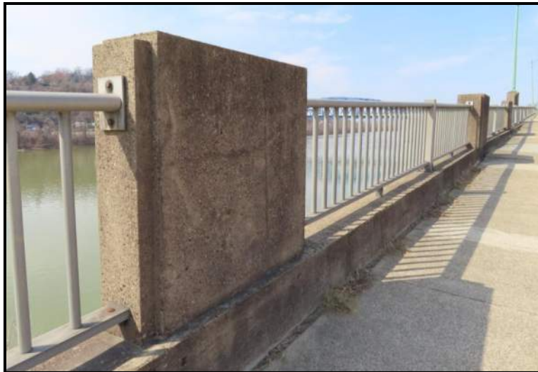
Typ. Concrete Railing Post. Example is at the South/Downstream East End. View WNW (WVDOH 3-13-2025)
