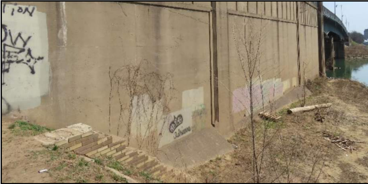
APE 1 – Stepped Feature 1 – This feature is at the lower left corner of this image. It is not very wide but appears to be a stairway access between grades at west abutment (downstream side). It appears to be unrelated to the original bridge construction. It perhaps is a utilitarian access installed for bridge inspections/maintenance.
