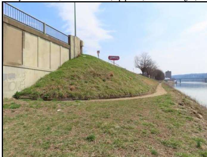
River Walkway, termination at bridge wingwall at east wingwall of bridge. View SE (WVDOH 3-13-2025). The same riverwalk termination occurs at the west wingwall as well.
