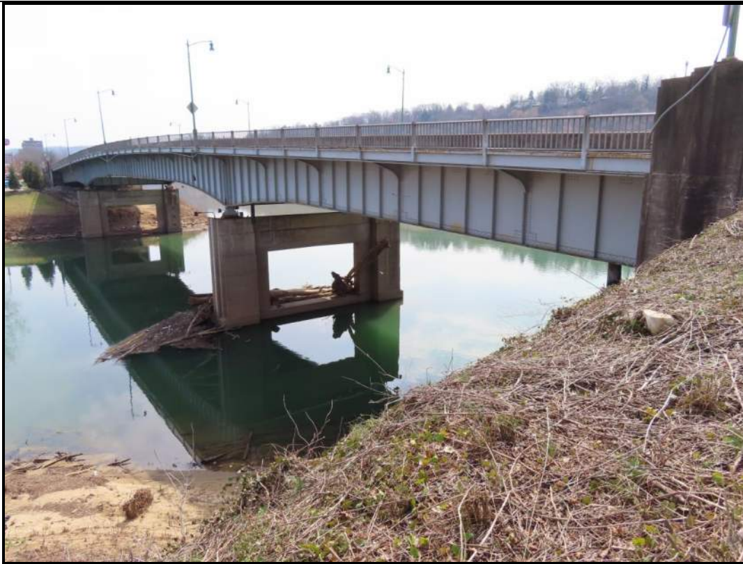
North/Upstream Elevation & Underside of Main Span. View SSE, taken from west bank of Elk River, at Union Square office complex. (WVDOH 3-13-2025)
