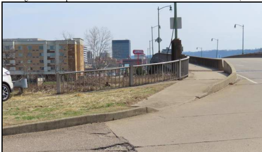
End of Railing at North/Upstream Side, West End; at Union Square Office Complex Entry (formerly Columbia Ave). View SE (WVDOH 3-13-2025).
