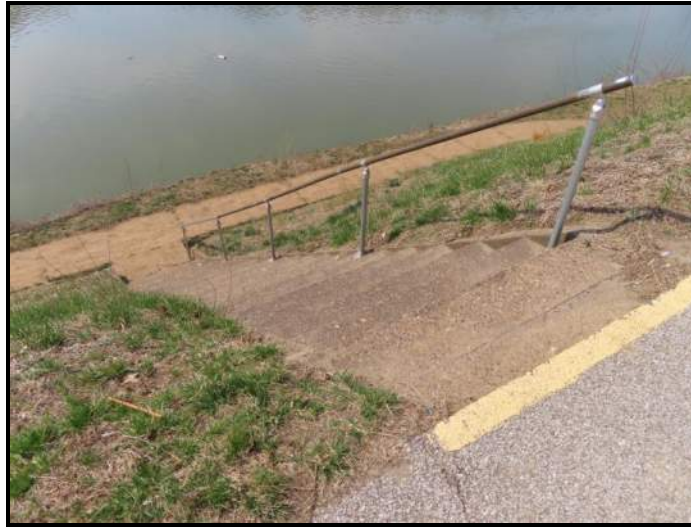
Typ. Staircase to River Walkway, located about 30 east of the south/downstream east wingwall. View SW (WVDOH 3-13-2025)
