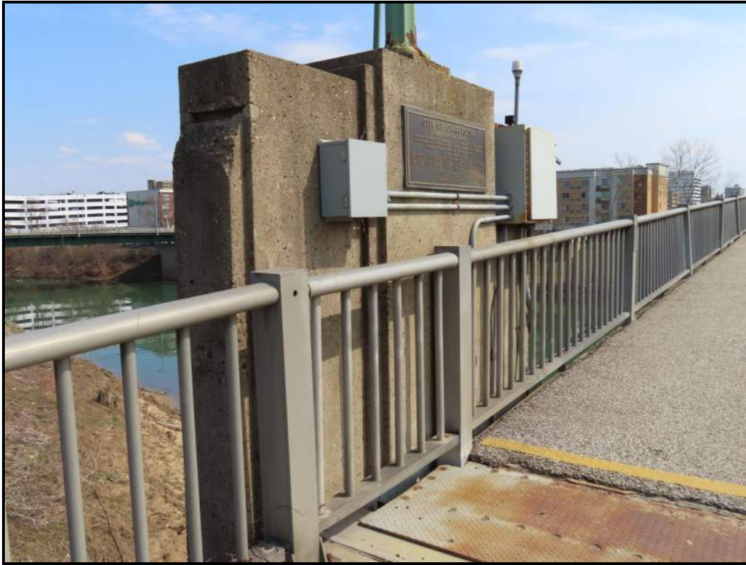
Pylon at West End, North/Upstream Side. Includes a 1980s plaque. View SE (WVDOH 3-13-2025)
