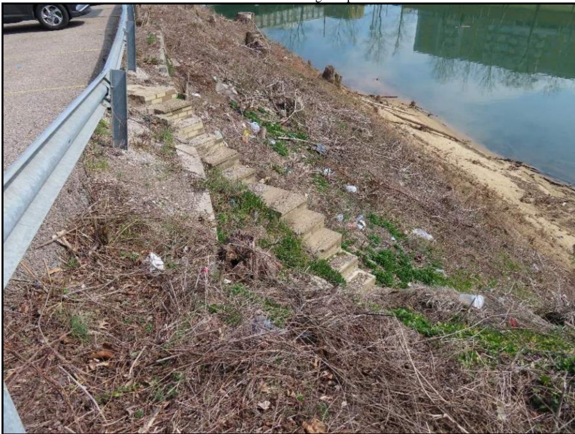
APE 1 – Stepped Feature 2 – this feature has is of the same design as Stepped Feature 1 above and appears unrelated to the original bridge construction. It is located off the Union Square parking lot (formerly Columbia Ave), and provides access to the lower grade at the west abutment (upstream side).
