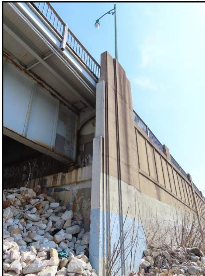
Typical Abutment Pylon. This is the pylon at the south/downstream side of the east abutment. View E (WVDOH 3-13-2025)
