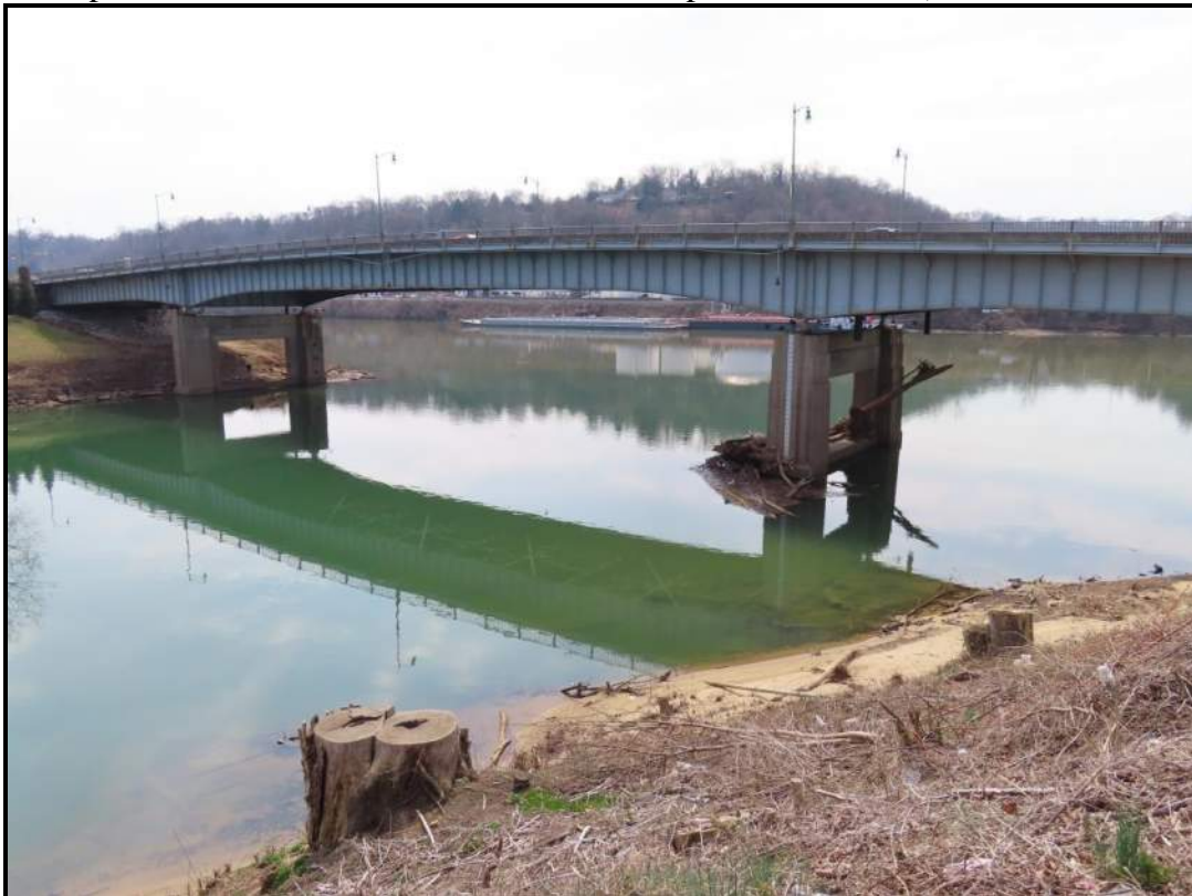
North/Upstream Elevation & Underside of Main Span. View SSE, taken from west bank of Elk River, at Union Square office complex. (WVDOH 3-13-2025)
