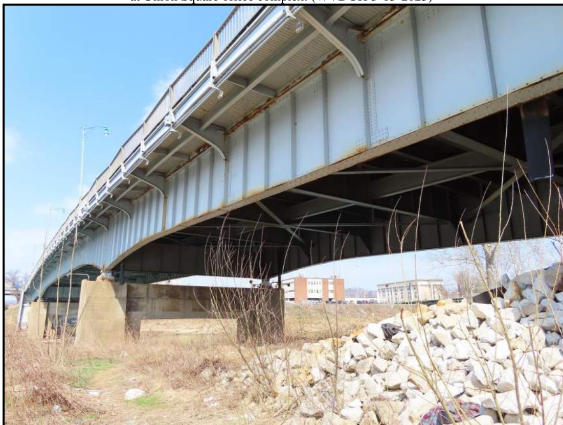
South/Downstream Elev. View NW, taken from east bank/confluence of Elk & Kanawha rivers (WVDOH 3-13-2025).
